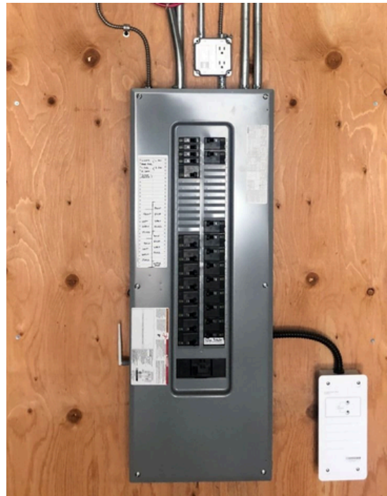
Electrical Panel with 240V electricity + breakers
