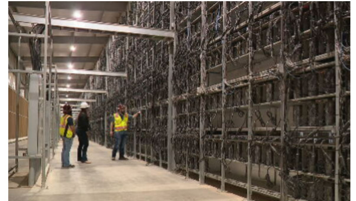
300 Megawatt Industrial Mine
